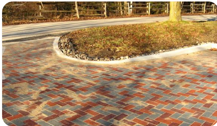
Eco-Flex Churchill pavers used for a parking lot pilot project at Kortright Centre for Conservation in Vaughan, Ontario
